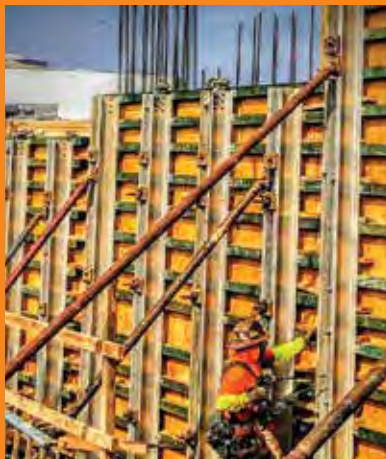
AS THE AUDITORIUM IS BEING BUILT , workers are tasked with many different jobs, like building the framework. Photo: Clemente Ortiz
